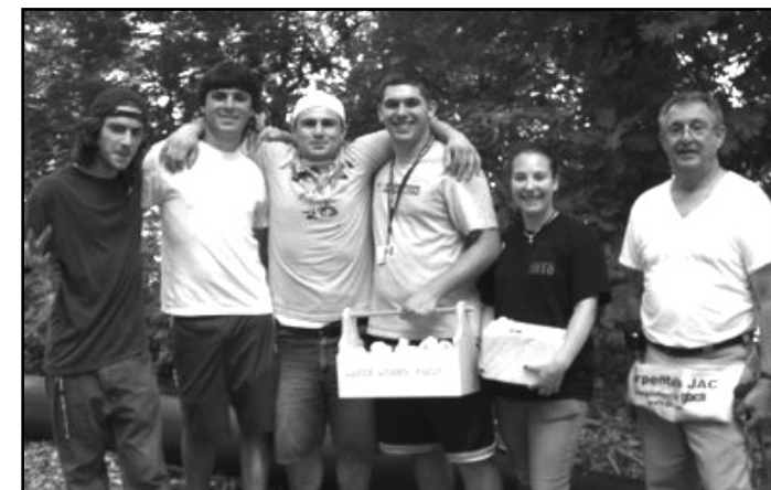
Marc teaches Arcadia University students how to install gutters to be used for rain collection.
